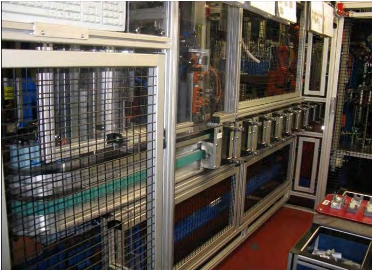
LFS-LAT Conveyor System
