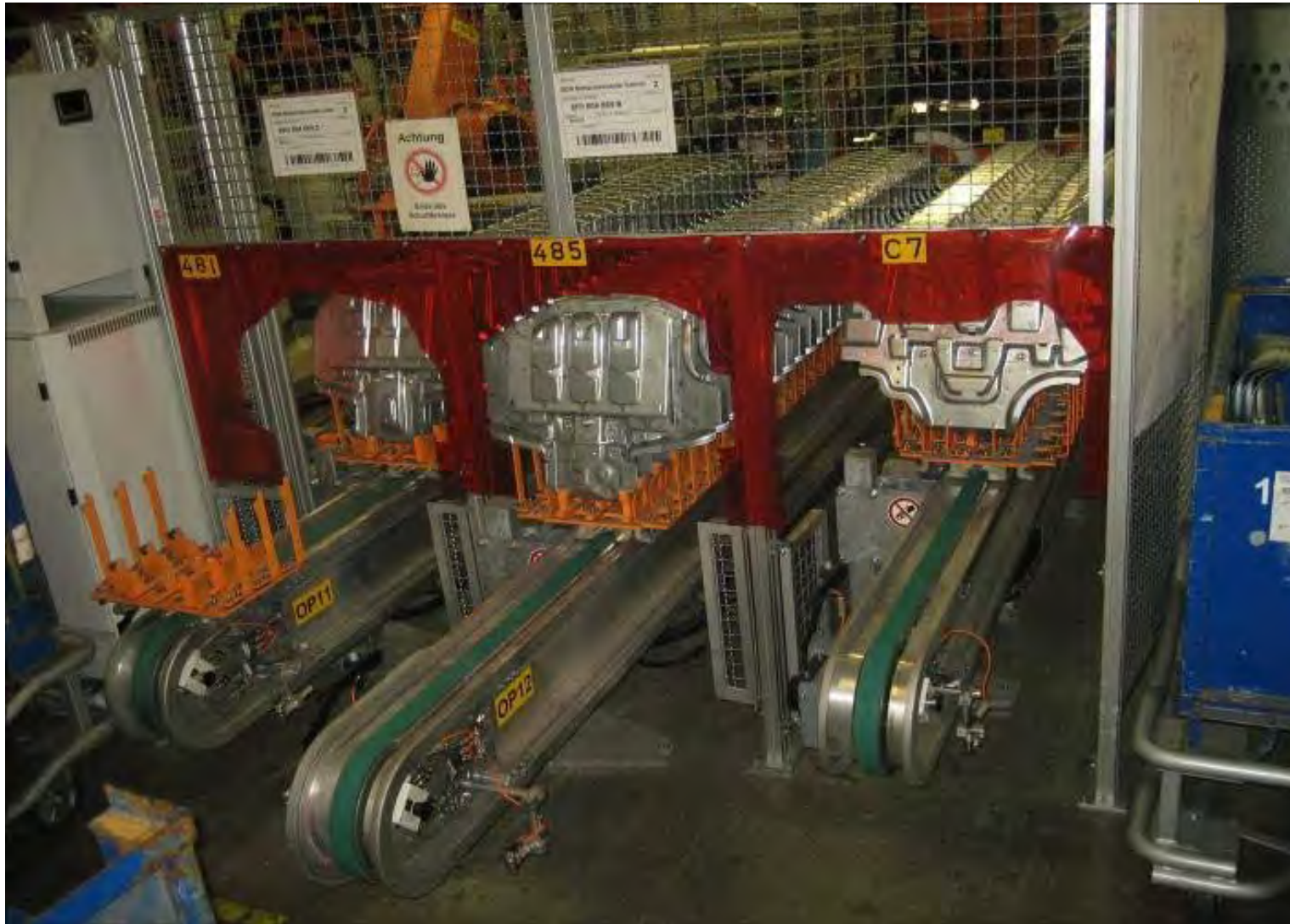
LFS-LAT Conveyor System
